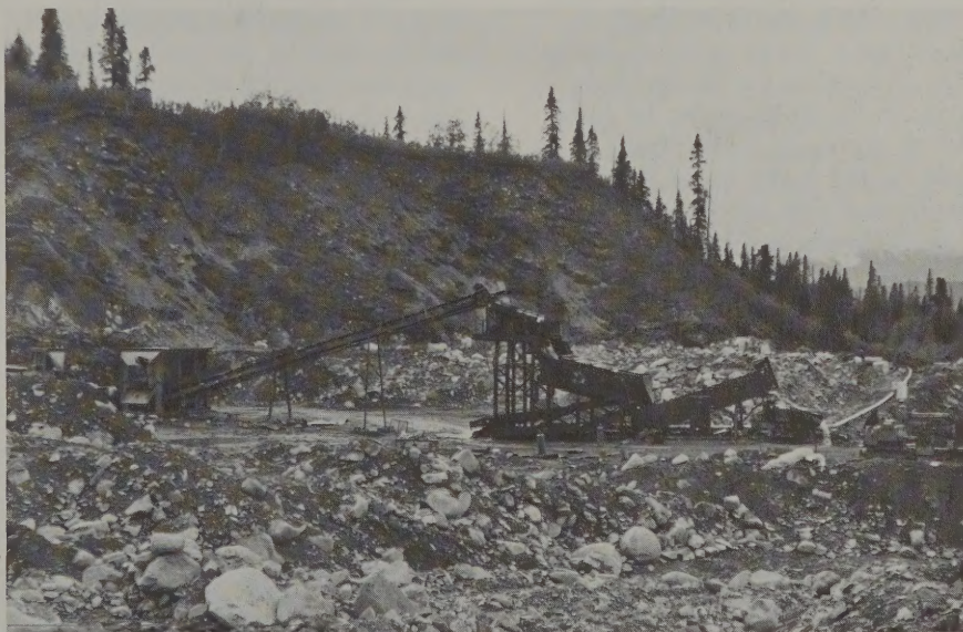
In this commercial placer mining operation on a gravel deposit in Alaska, the material is conveyed to a series of riffles designed to separate particles of gold from sand and gravel.
